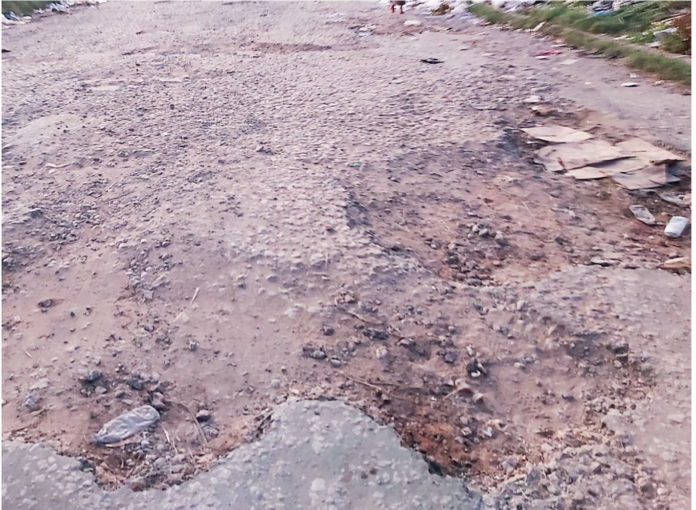
Roads with potholes show the reality of Pemba
